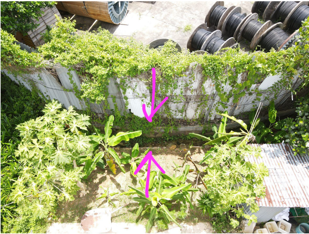
View B. Underground pipe and Existing 1m x 1m open channel (inaccessible area)
